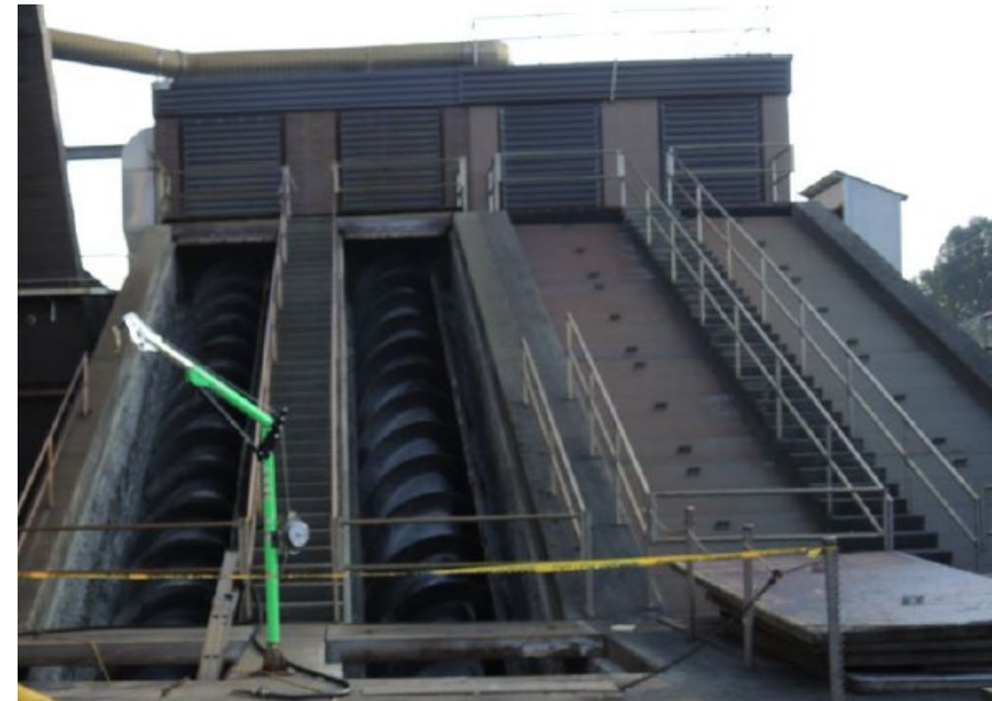
Influent Screw Pumps
