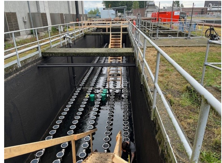
Solids Contact Tank Diffusers
