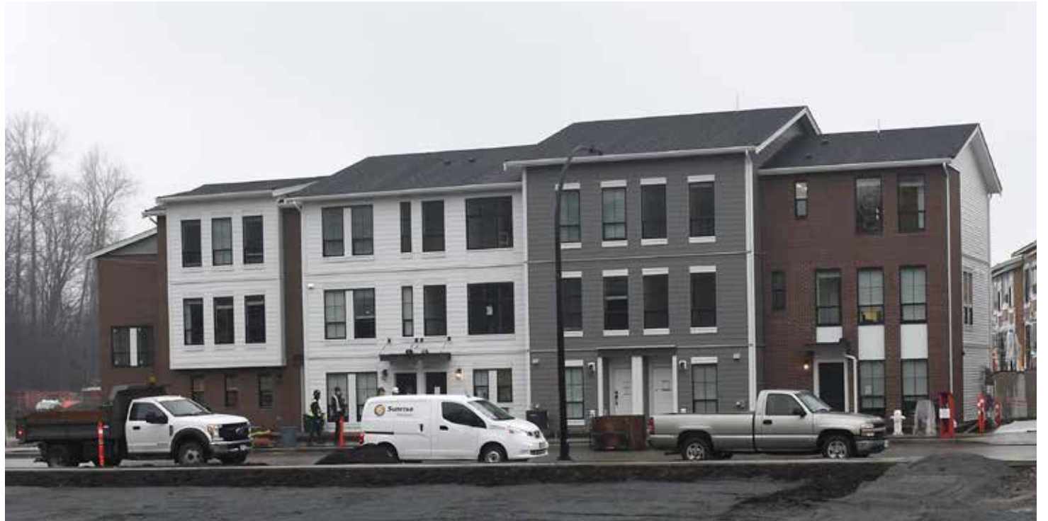
Construction is well underway for the first phase of the Rail District in historic downtown Abbotsford. (John Morrow/Abbotsford News)
