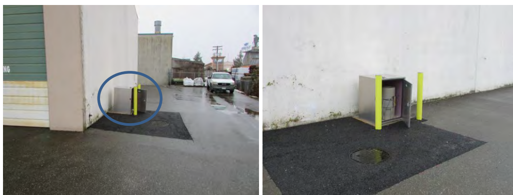
Figure 3. Photographs of a Sampling Kiosk at a Metal Finishers Strata Property
