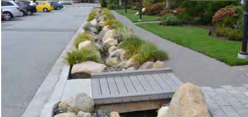
There are many ways to incorporate raingardens into streets. Adjacent land use, aesthetic and character, and context needs to be considered. Images: (middle) Centre for Neighbourhood Technology, (bottom) waterbucket.ca
